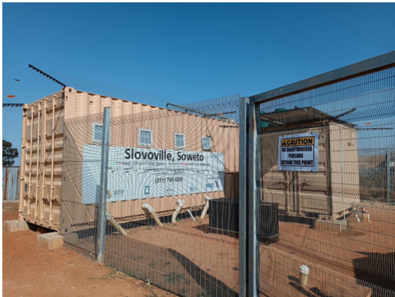
Non-Sewered Sanitation (NSS) system in Johannesburg, South Africa. The system recycles water for flushing.
